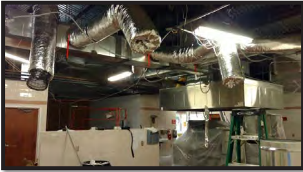
New A/C system in the kitchen at Ben Hill Griffin Jr. Elementary.
